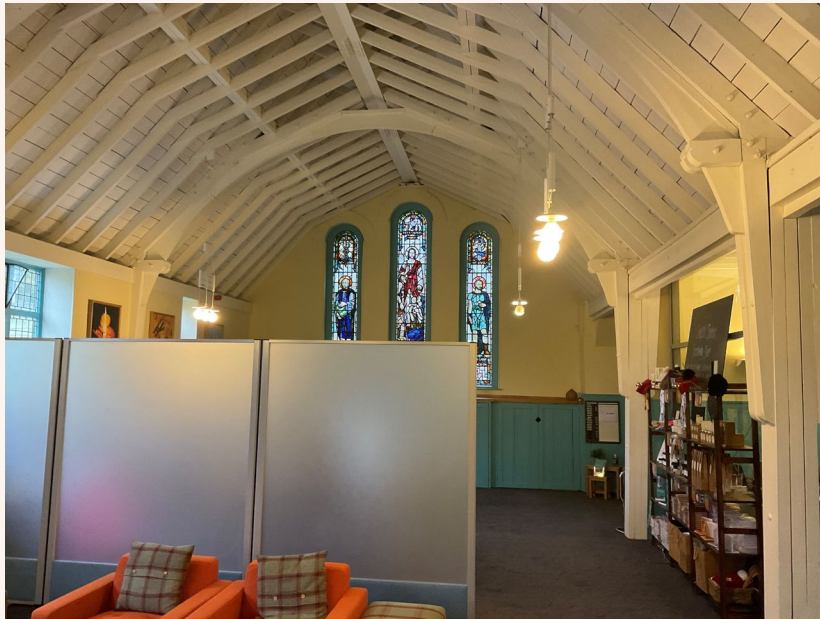
Looking to the North Interior view showing the wooden beams and columns holding the ceiling structure
