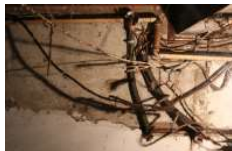
裸露的电线老化严重，会有安全隐患。 Exposed wires are aging badly, there will be security risks.
