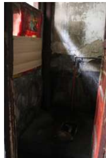
部分卫生间堆放杂物，使逼仄的空间进一步缩小，通风采光条件很差。Some restrooms piled up debris and cramped spaces, ventilation and lighting conditions are poor.
