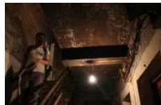
由于布局问题公共空间无自然日光，必须全天候借助人工照明，部分楼层无照明，部分楼层由居民合资购买了声控灯。Because of the layout, there is no natural daylight in the public space. It is necessary to use artificial lighting all day long. Some floors don't have lighting facilities, and some floors have sound control lights.
