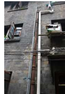
排污管道生锈腐蚀，部分管道已被弃用，部分管道由居民自行修补。无燃气管道，居民需要自行购买液化气罐。Some pipelines have been abandoned, and some pipes were repaired by residents themselves. Without gas pipelines, residents need to buy liquefied gas tanks themselves.
