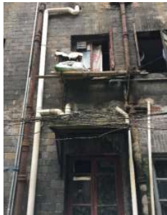
墙体外立面污渍斑斑，墙角野草苔藓丛生。The exterior of the wall is dirty and stained with weeds and moss in the corner.
