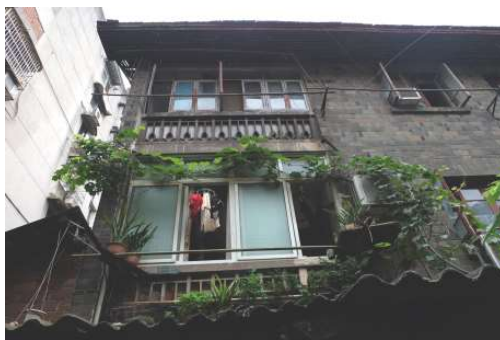
背立面花格栅栏杆 the Flower Grille Railings in the Back Elevation
