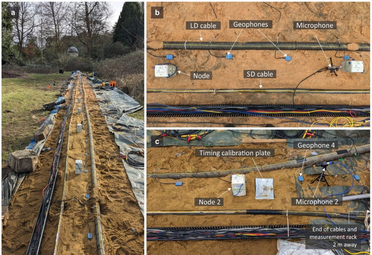
Fig. 3. (a) View of the test bed from the MR end. For many of the testing sessions, the ground was saturated due to considerable precipitation in preceding days. (b) Close-up photo of cables and seismic and acoustic sensors. (c) Location of the timing calibration plate near node 2, close to the MR end of the cables. Here the two submarine cables diverge slightly. Their ends are just off the picture, extending approximately a further metre in length.
