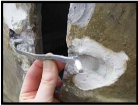
Old fixings and over-paint
